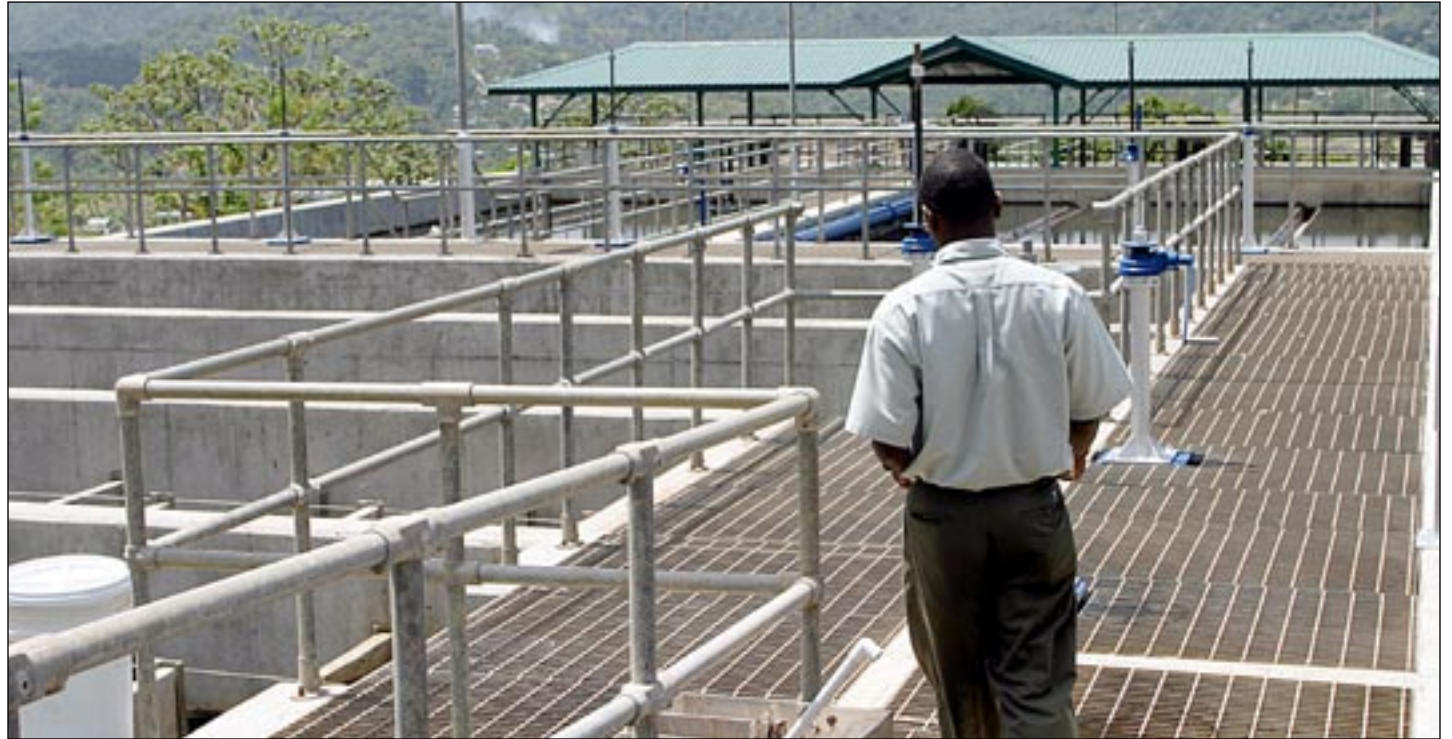
Ciceron Treatment Plant
