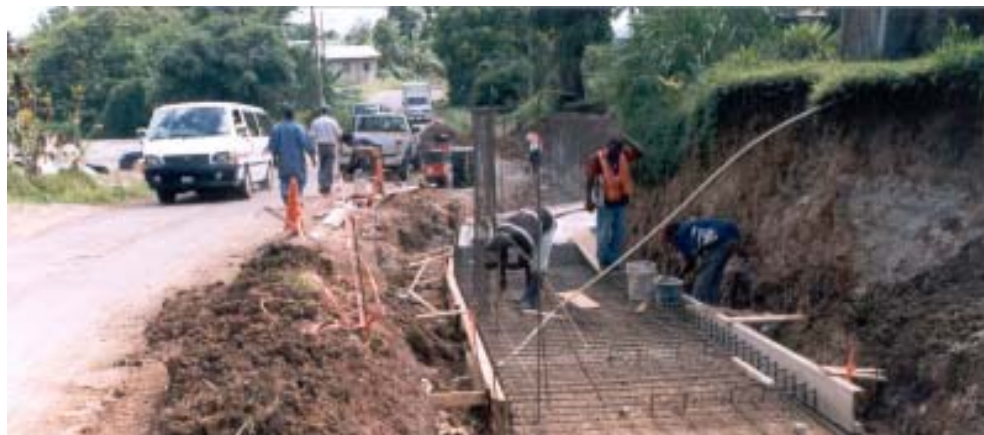
Road construction in the rural areas has taken on new dimensions in St. Lucia
