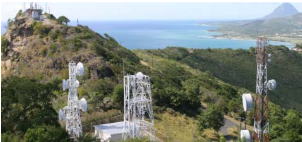
The expansion of telecommunications infrastructure.
