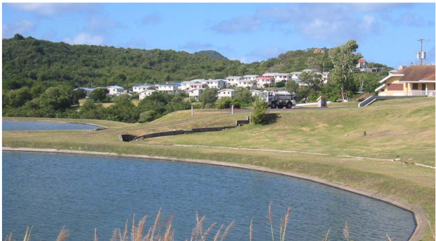
Appropriate treatment of liquid waste is being implemented by public and private sector agencies including WASCO.
