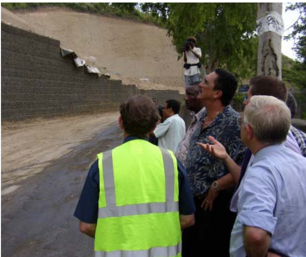
Project officials explain to Dr Anthony how a new earth retaining technology is allowing the widening of the road on the steep hill next to the Choiseul cemetery.
