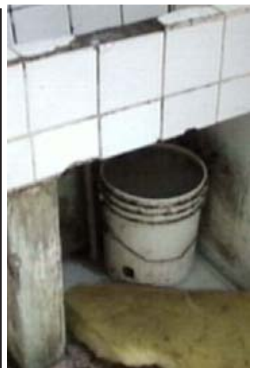
Part of the broken infrastructure of the old prisons
