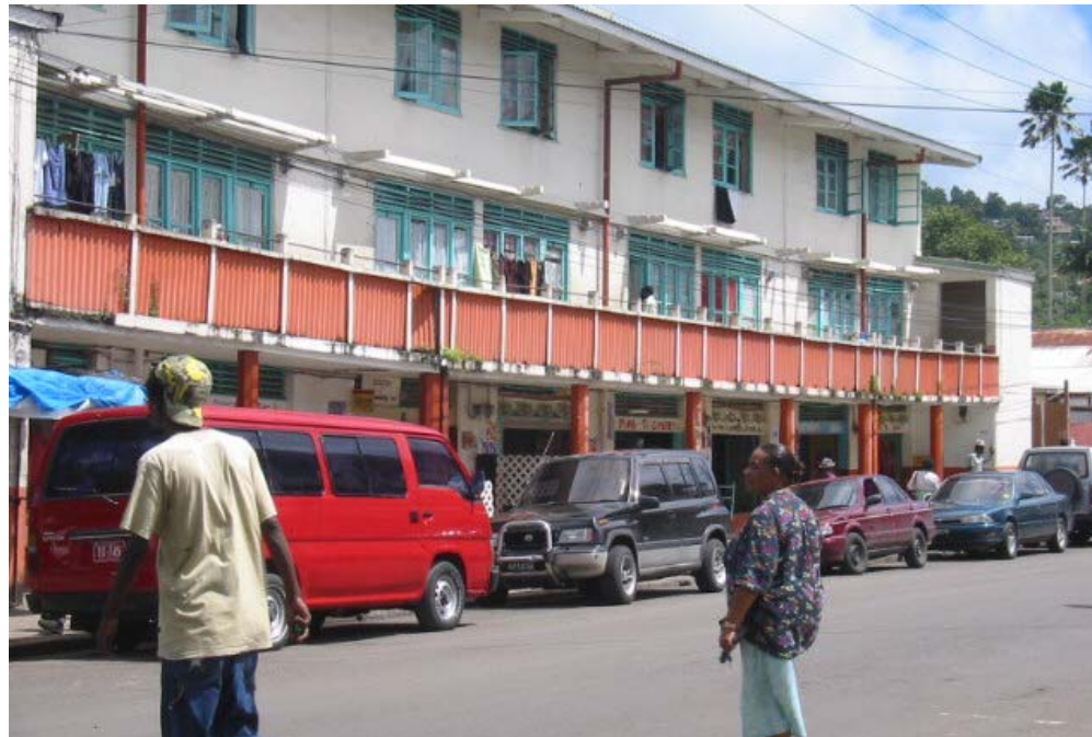
One of the CDC apartment blocks earmarked for replacement. Engineers have advised that these buildings are no longer safe.
