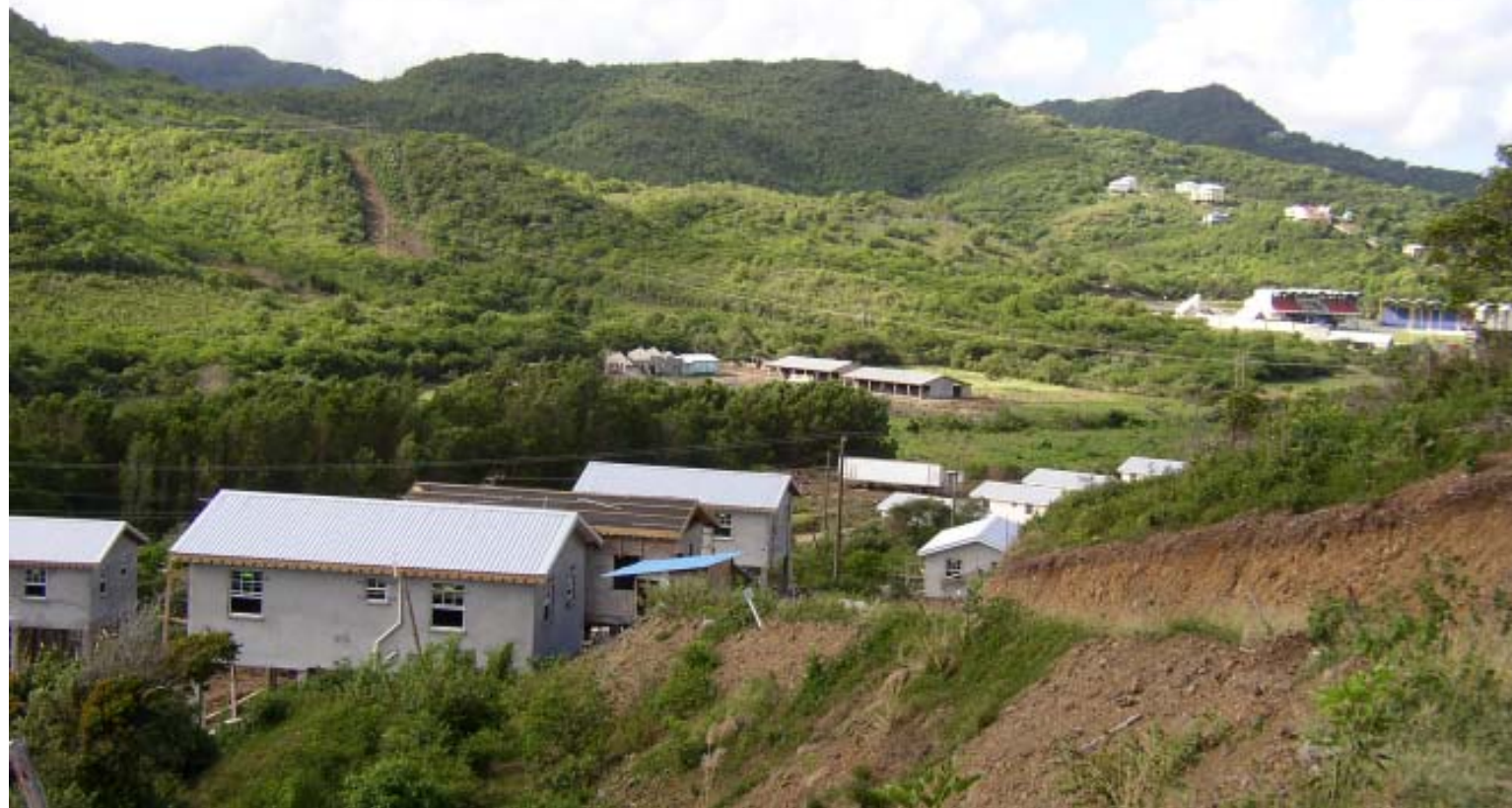
New houses under construction at the Beausejour development, for low income earners. The cricket ground in the background.
