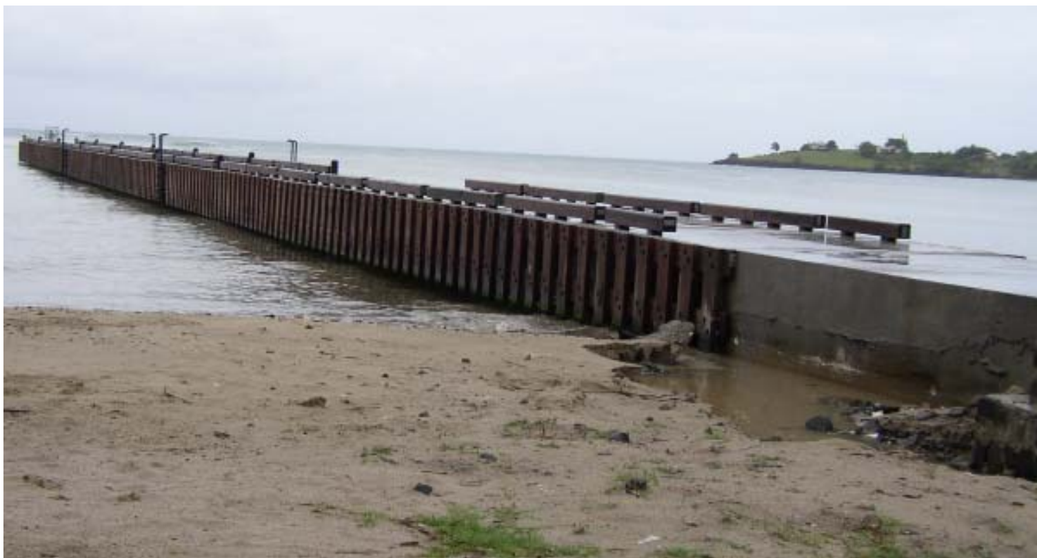
The new jetty in Laborie with potential to facilitate tourism and fishing activities.
