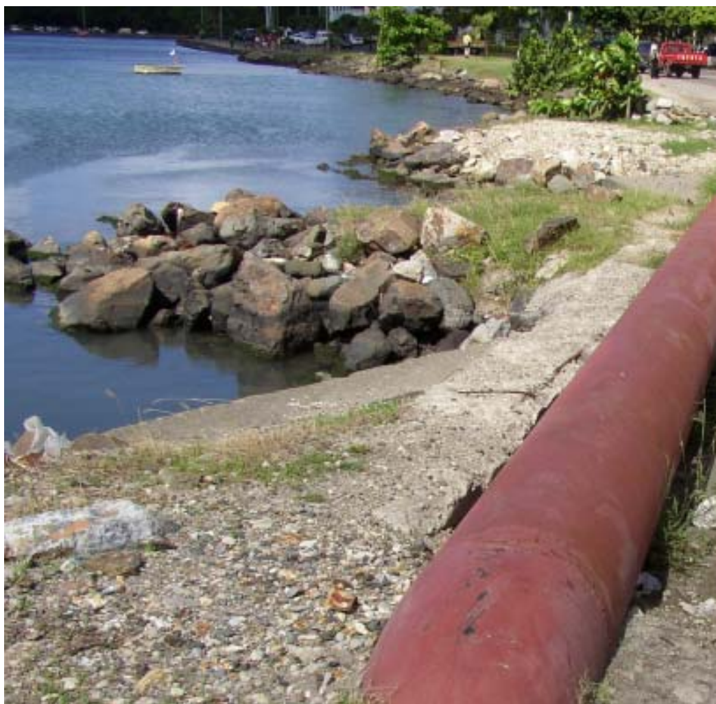
Part of the new 20 in. main along the Castries waterfront: water woes in the past
