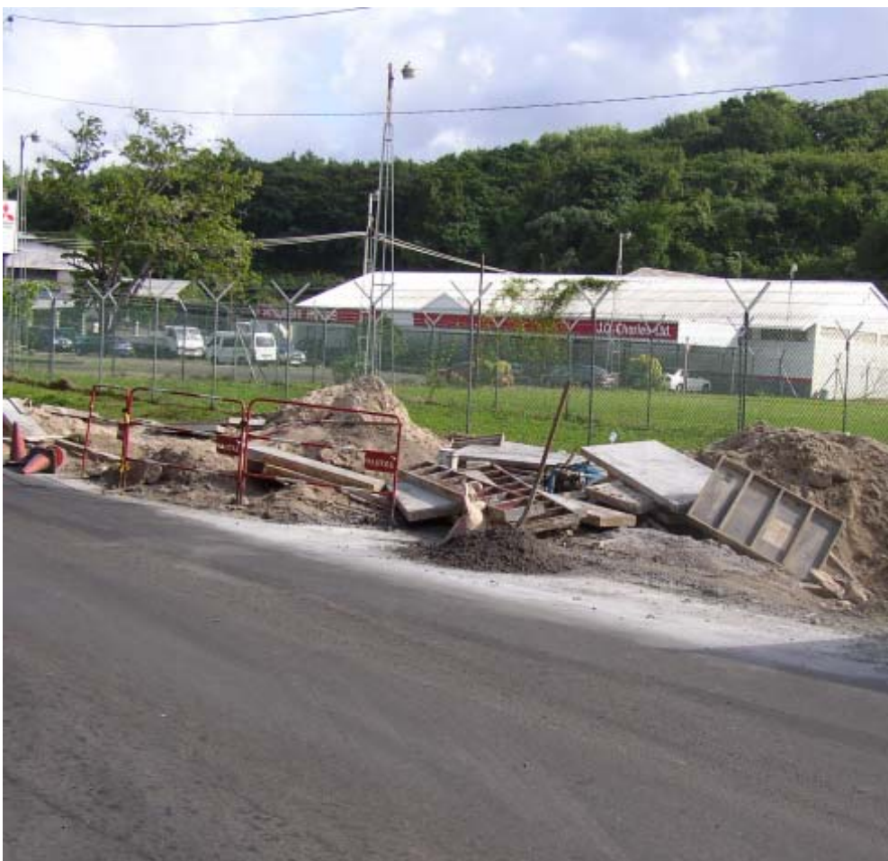
Construction activity during the laying of the twenty inch pipe has always been a source of curiosity for motorists, causing occasional delays in traffic flow.
